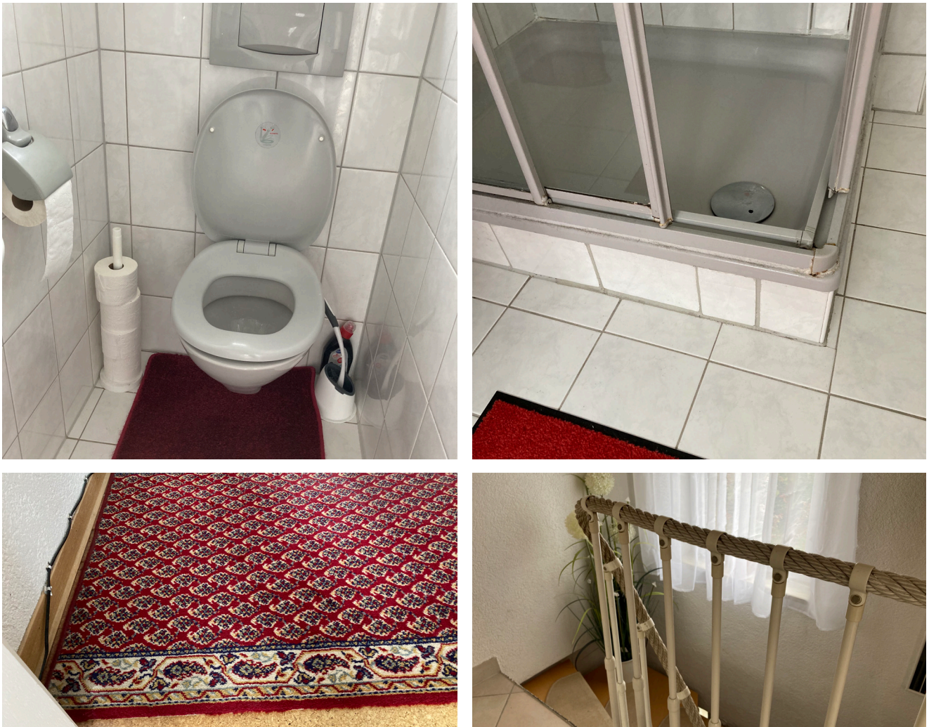
Figure 2. Typical fall hazards in an elderly home. Photo credit: Author's own
